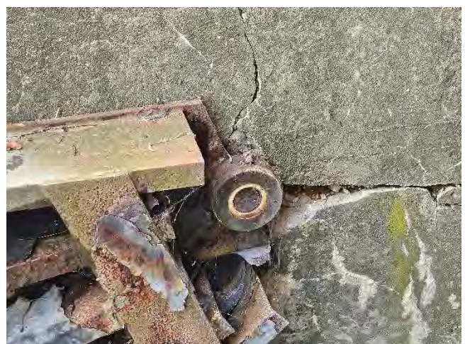
South Trunnion Structural / Radial Cracking
