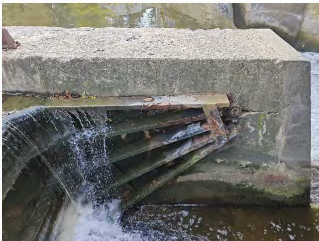
South Trunnion and Structural Deficiencies
