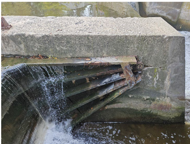
South Trunnion and Structural Deficiencies
