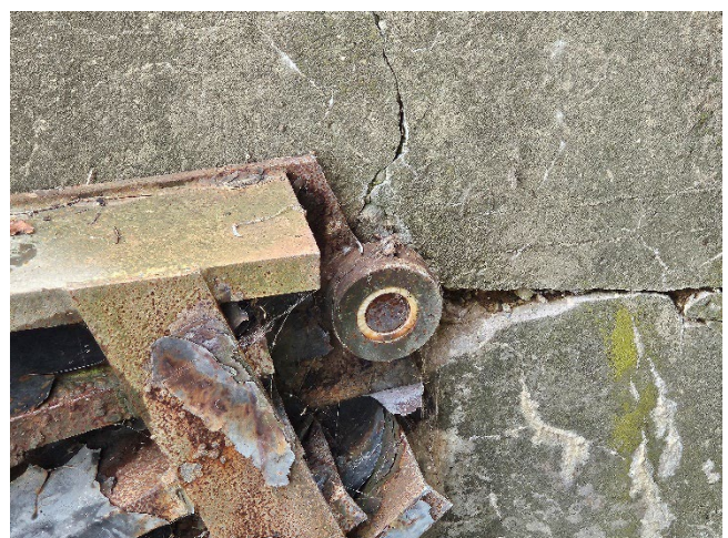
South Trunnion Structural / Radial Cracking
