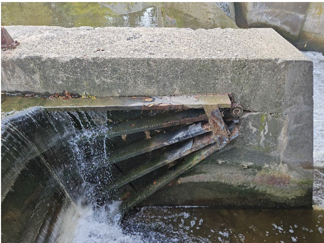
South Trunnion and Structural Deficiencies
